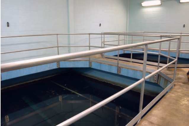
Water System Filtration Tank
